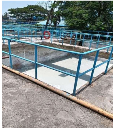
Fig No.1 Sewage treatment plant
