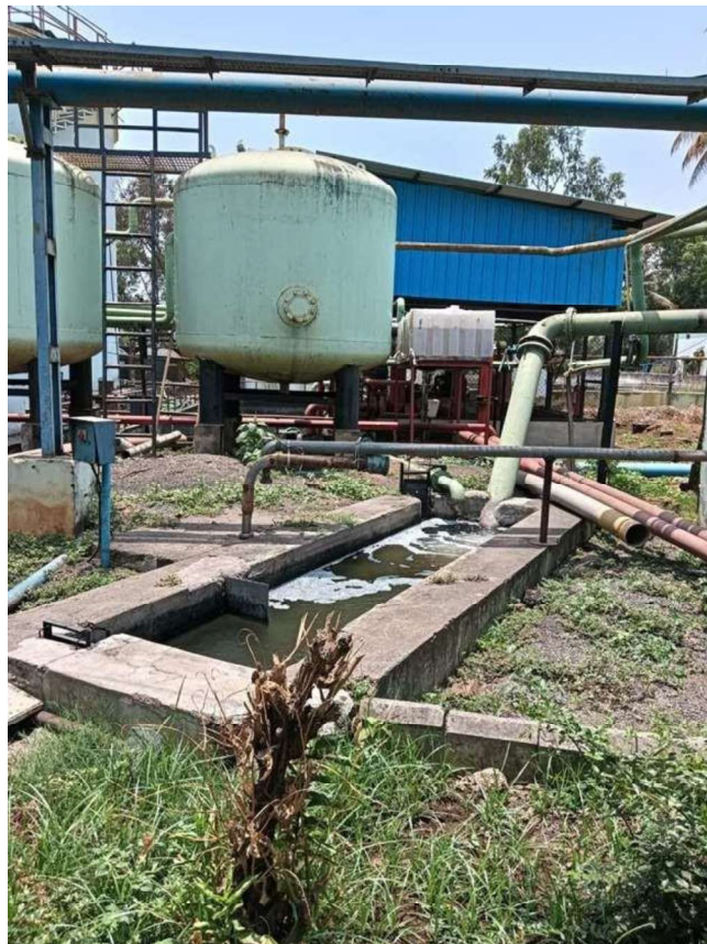
Fig no. 2 Effluent treatment plant
