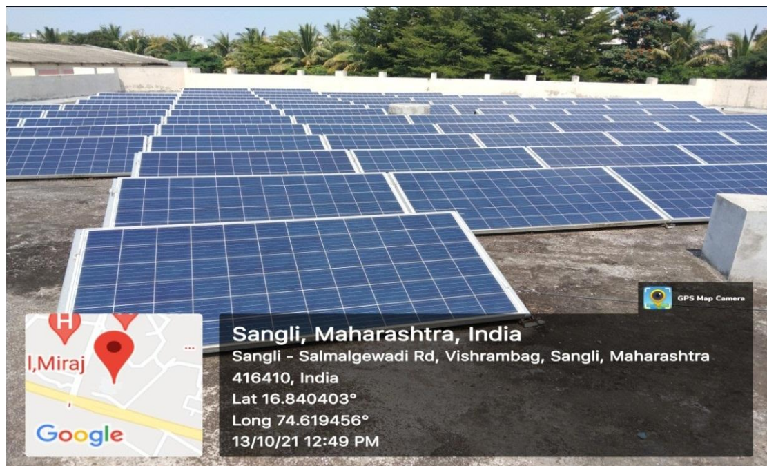
Plate No.21: Solar Photovoltaic Application at VPIMSR, Sangli
