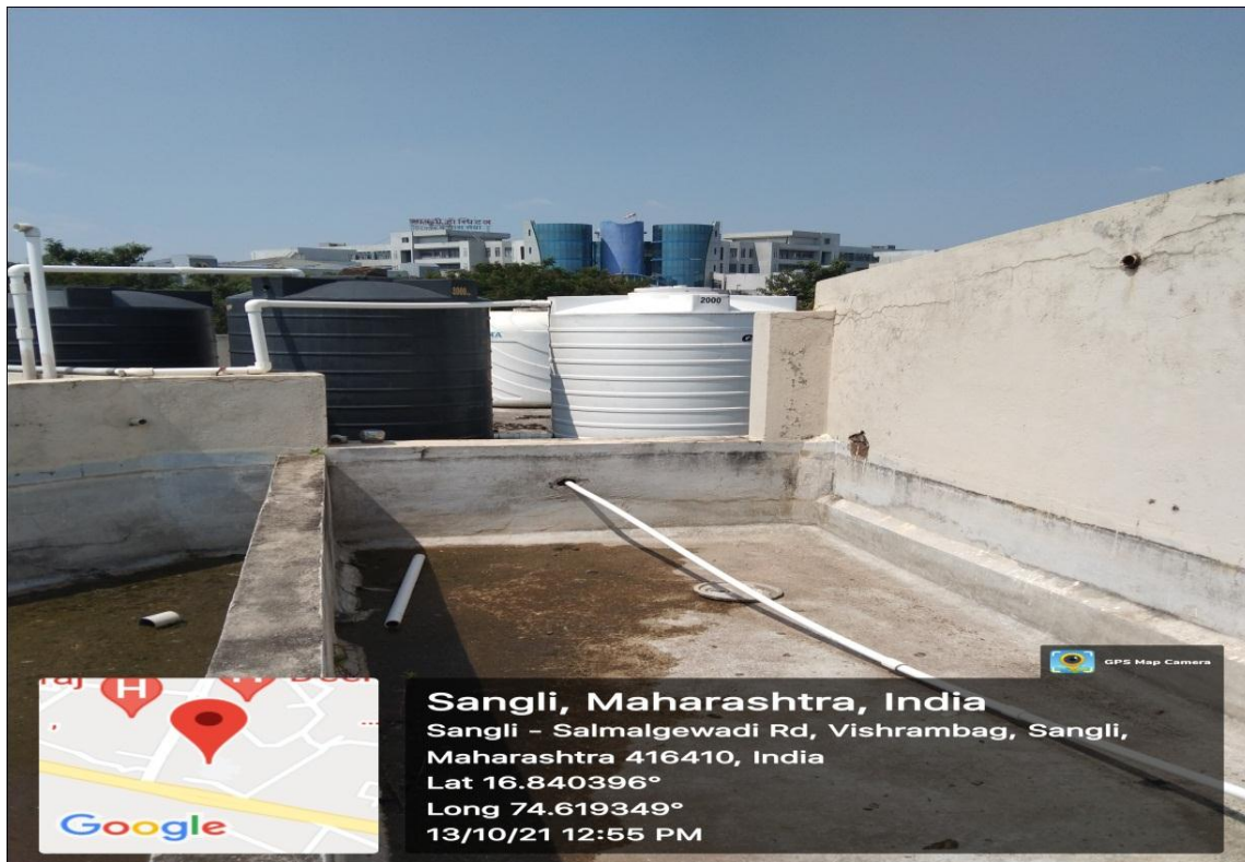
Plate No.24 : Rain water collection and storage at VPIMSR, Sangli
