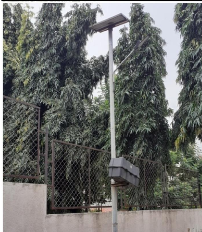
Plate No.21 C: Solar Street lamp installed at CSIBER, Premises
