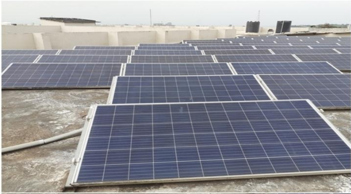
Plate No. 21: Solar Photovoltaic Application at CSIBER Institute, Kolhapur.
