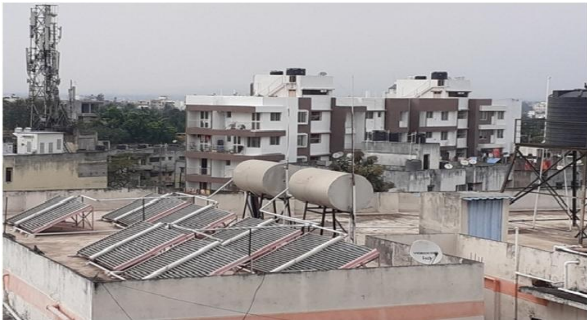
Plate No. 21 A: Solar Photovoltaic Application at CSIBER Institute, Kolhapur.
