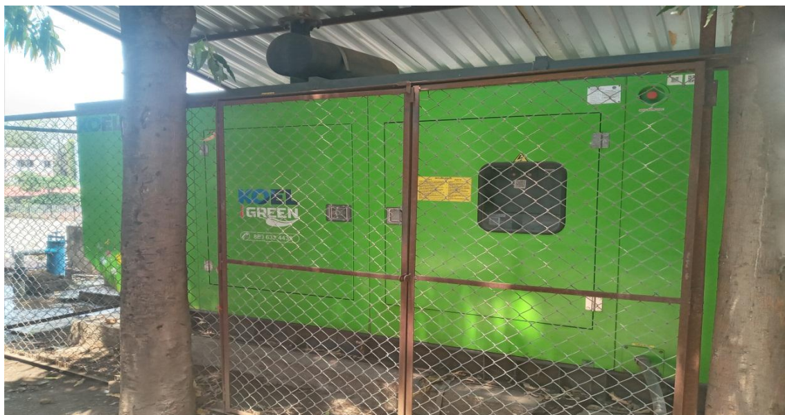
Plate No. 19: Green Power Generator operated on Diesel at Institute campus.
